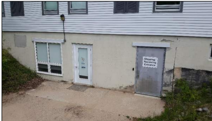
Photograph 9: Concrete foundation wall crack
