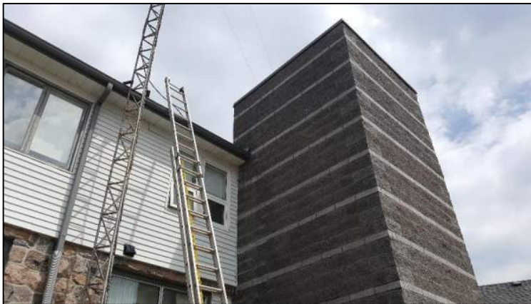
Photograph 6: Elevator exterior wall staining
